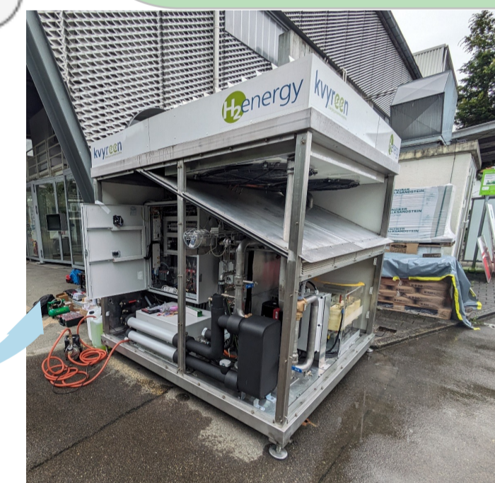
Fuel cell system (Kvyreen) installed at Empa.
